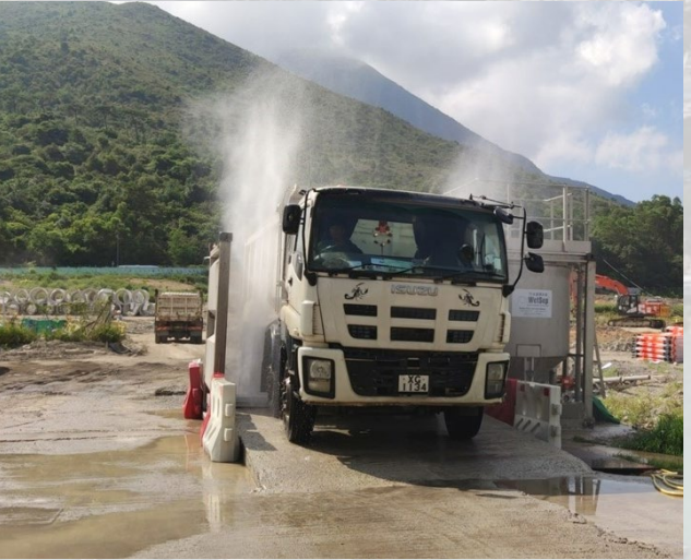
Wheel Washing Facility
