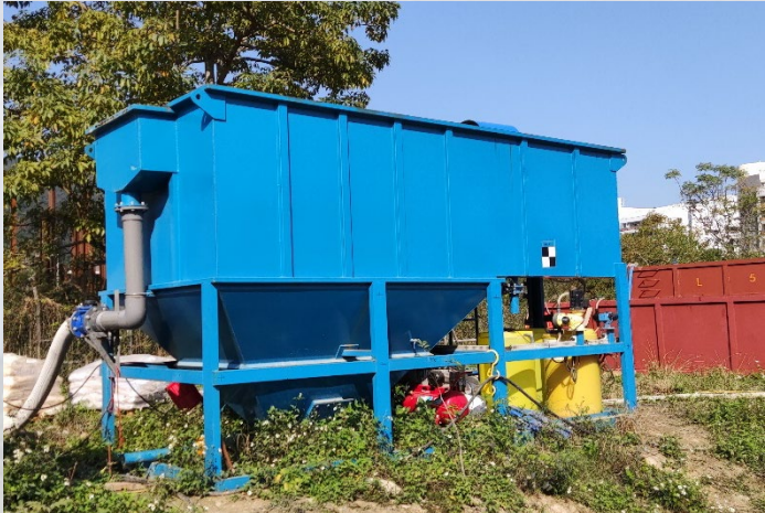
Wastewater Treatment Facility
