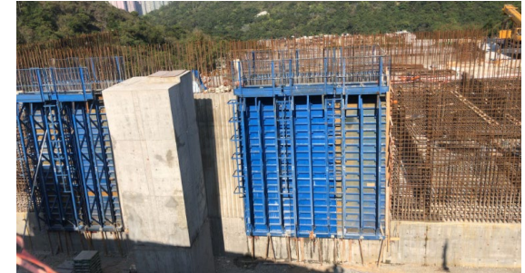
Salt Water Service Reservoir
